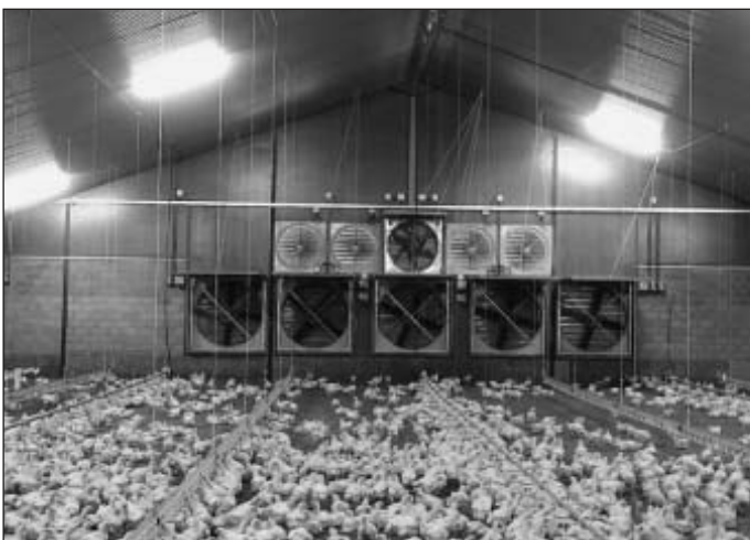
Fig. 1: With tunnel ventilation, the foul air is extracted at the front side (Photo Fancom)
