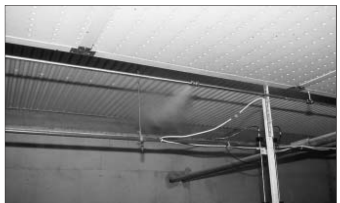
Fig. 3: Water atomiser facility beneath the fresh air duct in the stable
