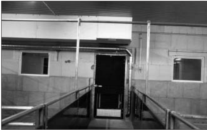
Fig. 2: Fresh air ducting through the feeding alley
