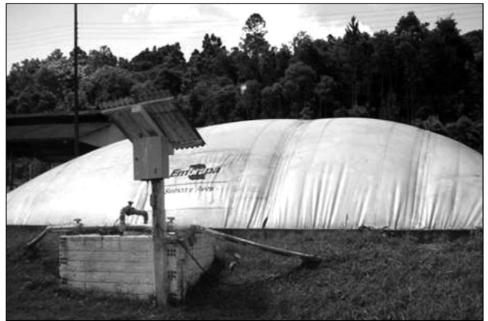
Fig.3: Biogas plant with solar-driven pump for circulation of the substrate
